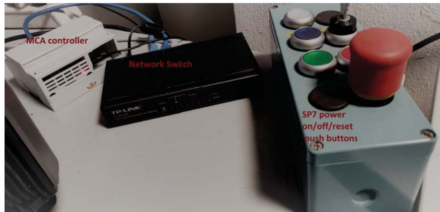
Figure 2.11 MCA controller connected to the Ethernet switch.
