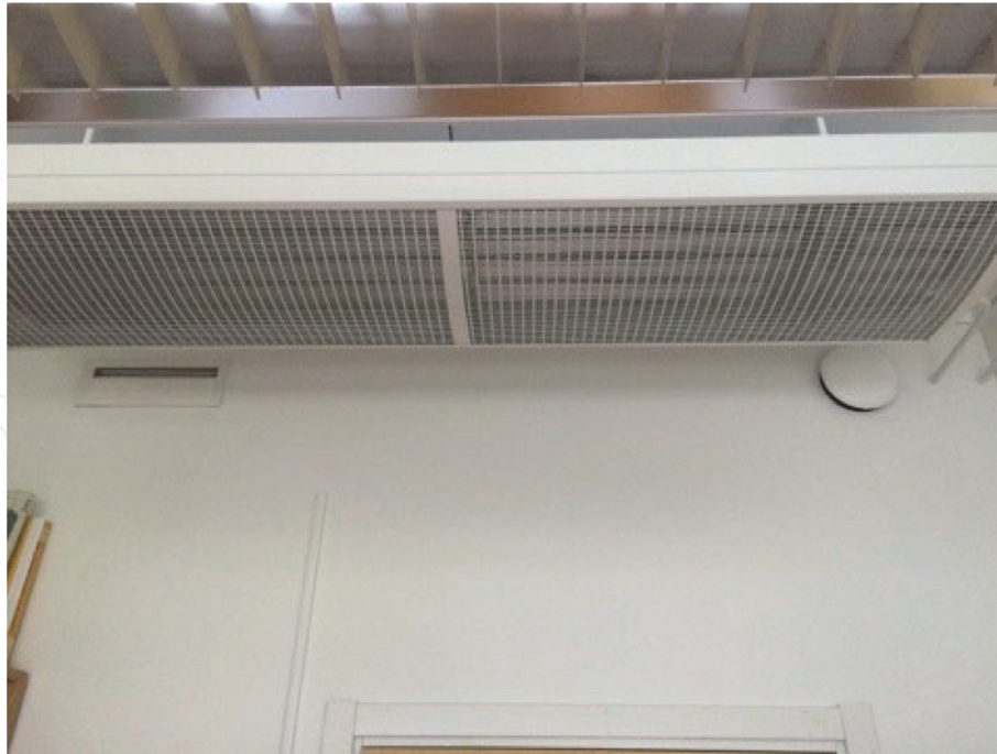
Figure 5. Retrofit of cooling beam (with attached light fixture) leading to a high degree of ventilation short-circuiting. Air supply device to the left and air exhaust to the right.
