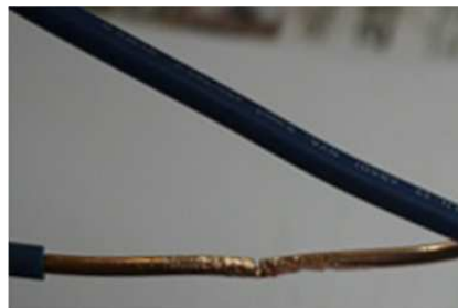
Figure 1. The damaged conductor
