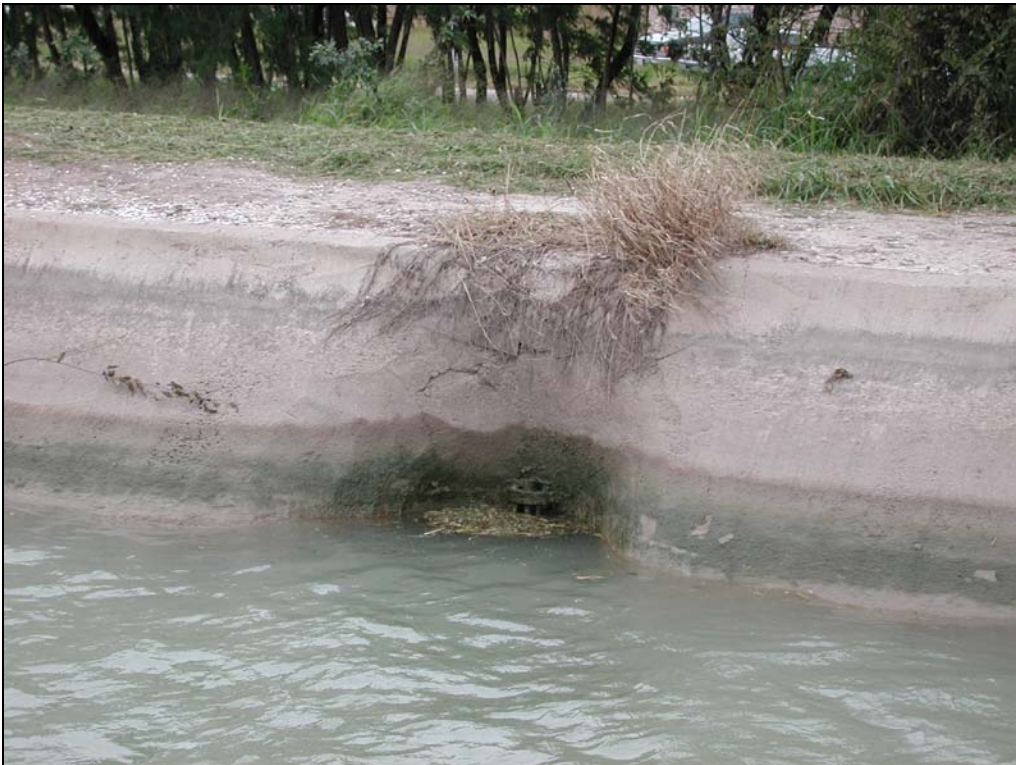
Figure 3d. Site 2 – an abandoned gate associated with the area of thick vegetation.
