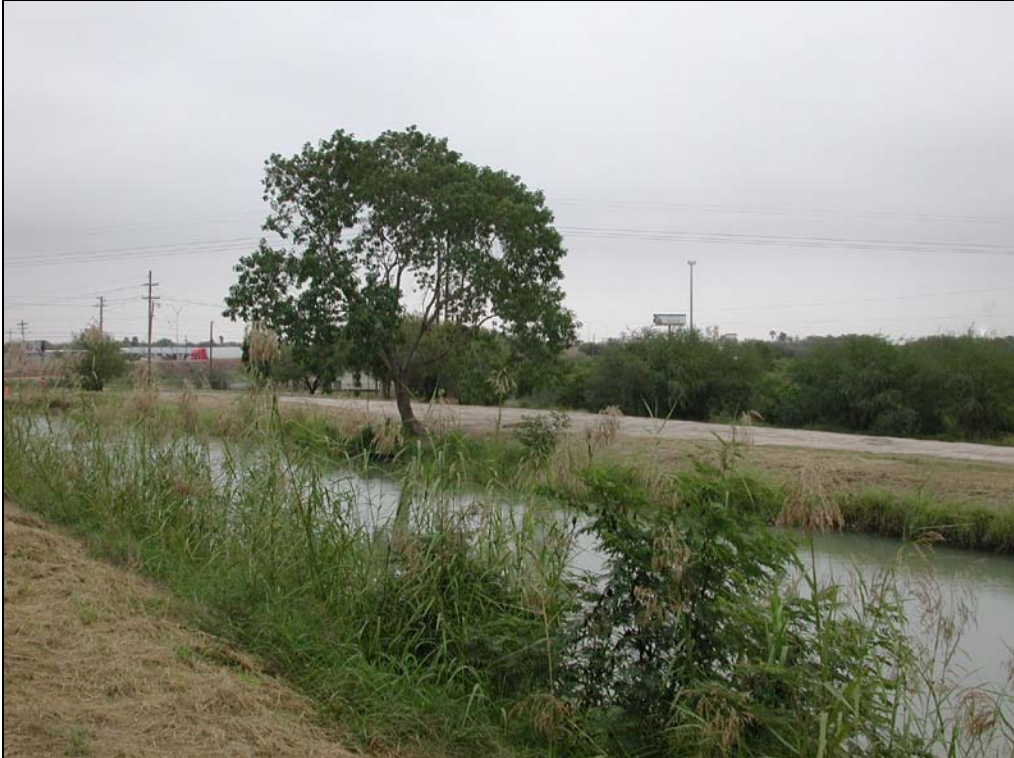
Figure 2c. Photograph of Site 1 – an unlined canal segment with a hole in the embankment.
