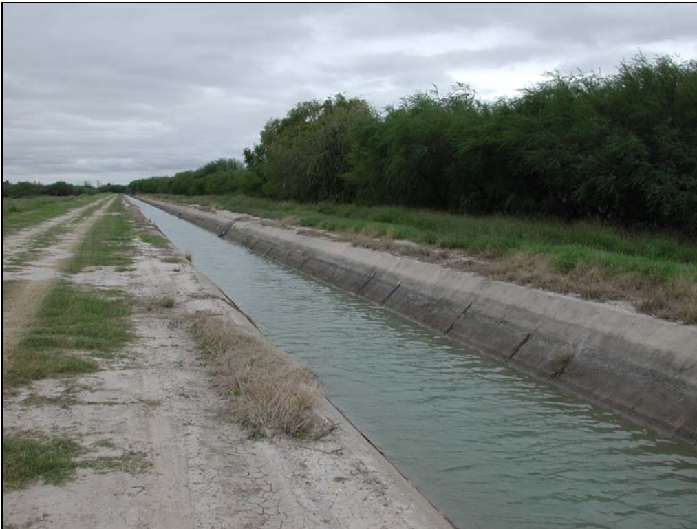
Figure 4c. Site 3 – showing cracks and thick vegetation on one side of the canal.
