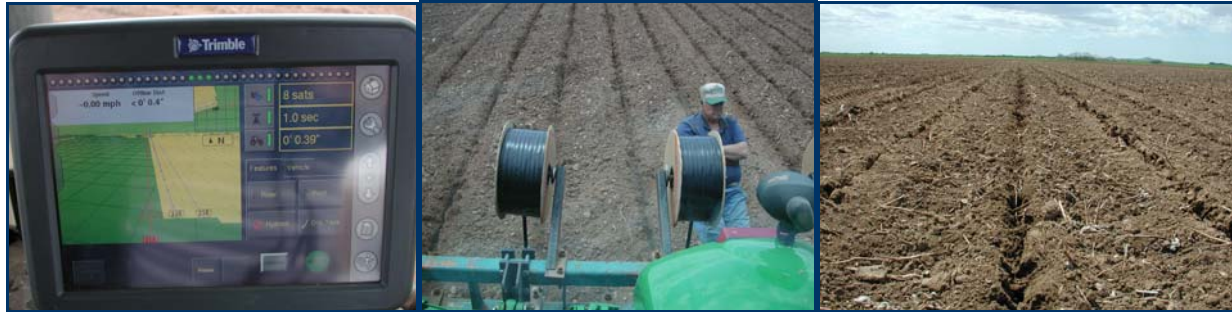
Figure 13. GPS Auto-steer technology was used to bury tapes 12 to 14 inches deep on 40-inch centers with sub-inch accuracy, Chillicothe, Texas, 2006. Left panel: GPS monitor; middle panel: installing drip tape; right panel: installed tape with sub-inch accuracy.
