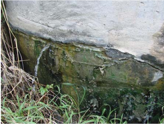
Figure 6. Leaking from standpipe
