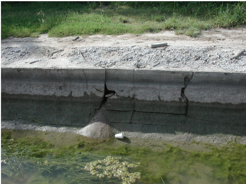
Figure 1. Large cracks and aquatic vegetation shown above contribute to higher total losses of canal segments.
