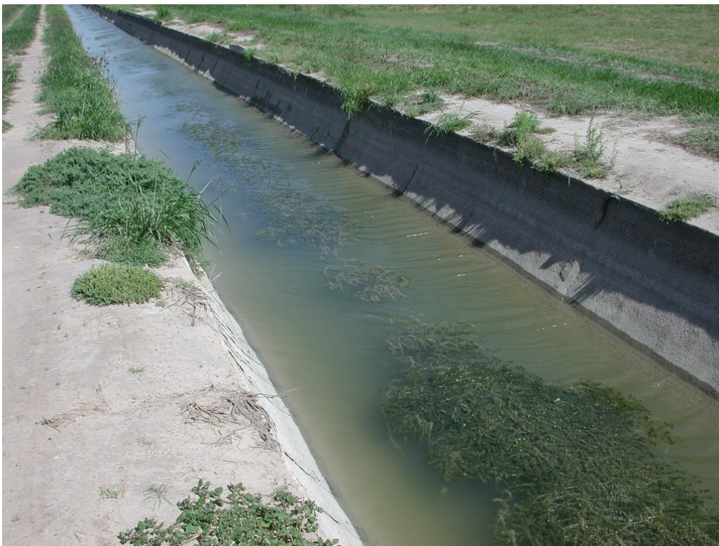
Figure 5. Photo of test segment UN1 showing aquatic vegetation problems.
