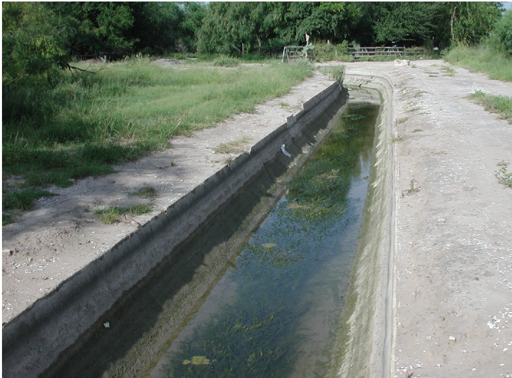
Figure 7. Photo of test segment UN2 showing aquatic vegetation problems.
