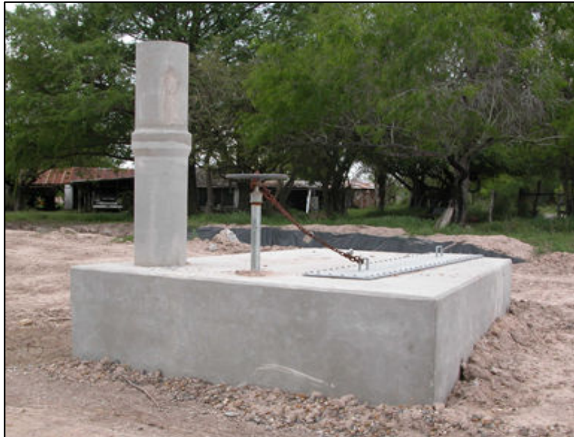
Figure 6. Showing an exposed box structure
