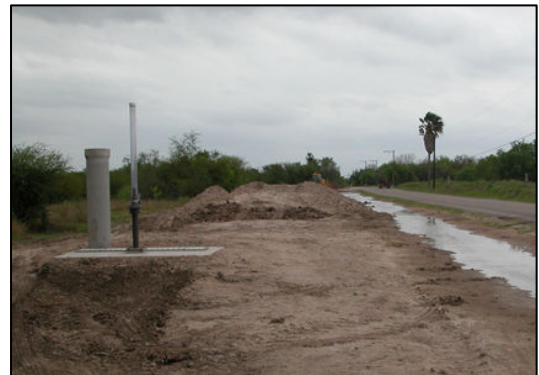
Figure 2. Visible leaks shown after construction
