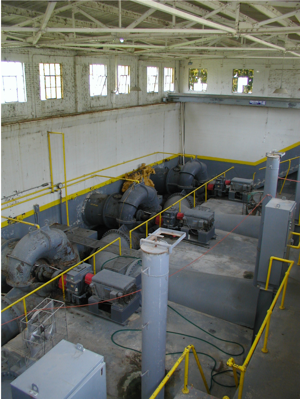
EXHIBIT C6. Delta Lake Irrigation District's Pumping Station and Pumps, 2003 (Wolfe).
