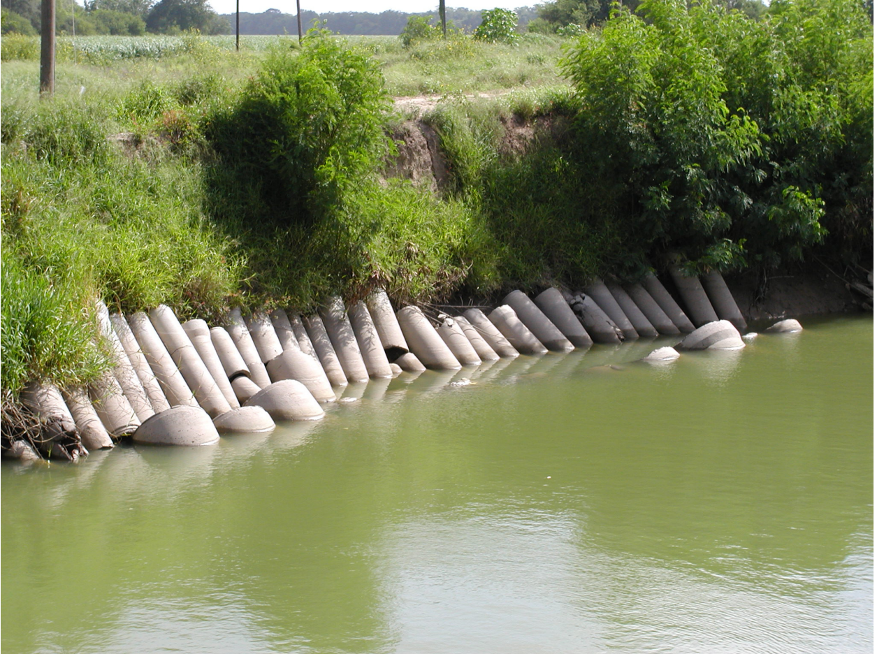
EXHIBIT C9. Delta Lake Irrigation District's Main Earthen Canal, with Concrete Pipes Placed Along the Bank to Lessen Soil/Bank Erosion, 2003 (Wolfe).
