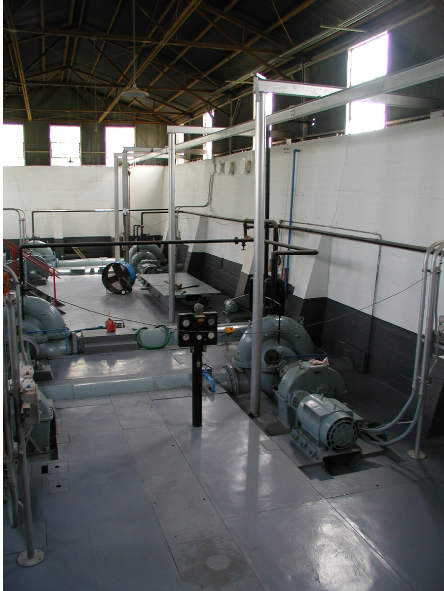
EXHIBIT C2. Harlingen Irrigation District Cameron County No. 1's Pumping Station and Pumps, 2003 (Wolfe).
