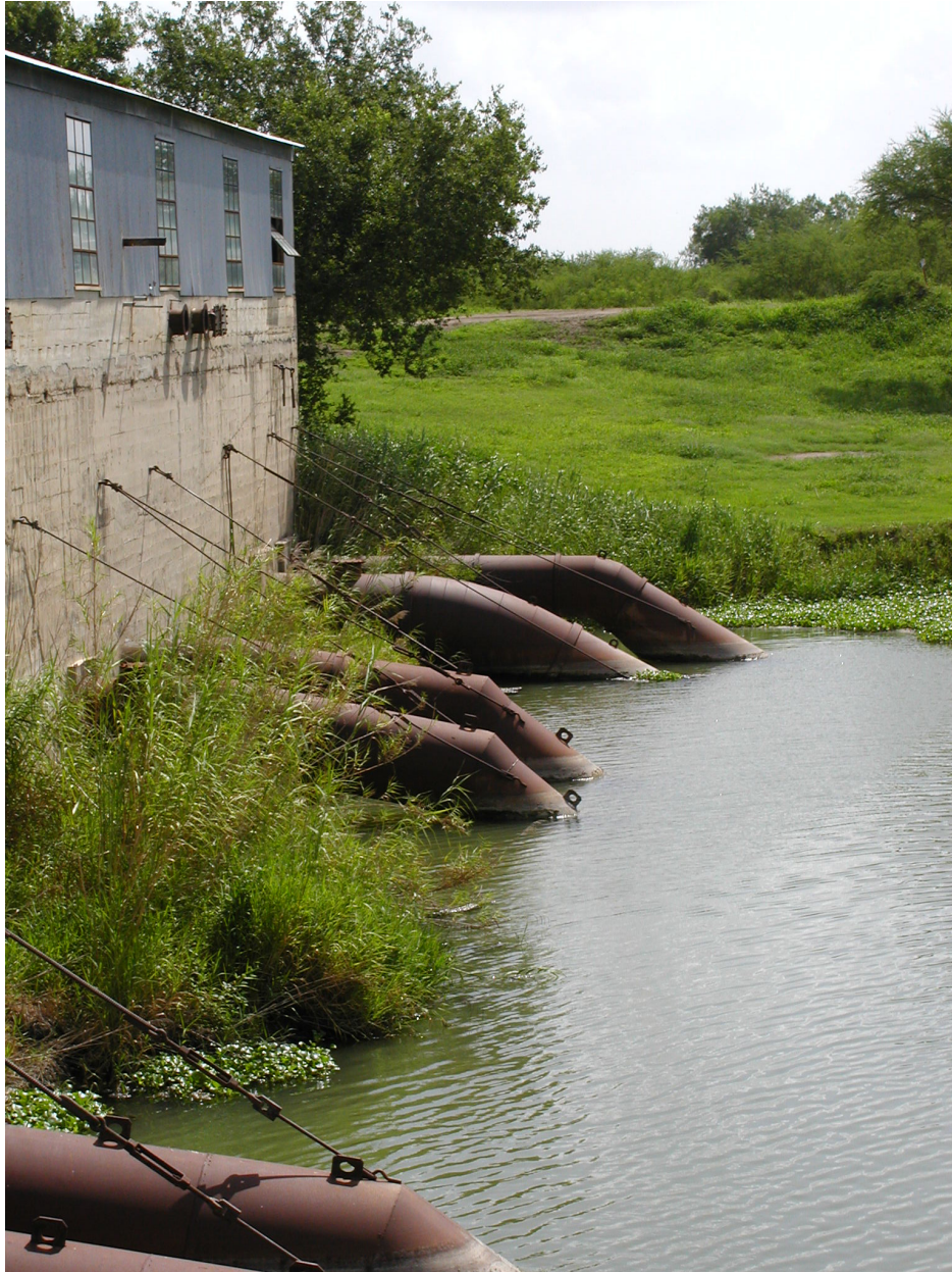
EXHIBIT C3. Rio Grande View of Harlingen Irrigation District Cameron County No. 1's Pumping Plant and 48-inch Inlet Pipes, 2003 (Wolfe).
