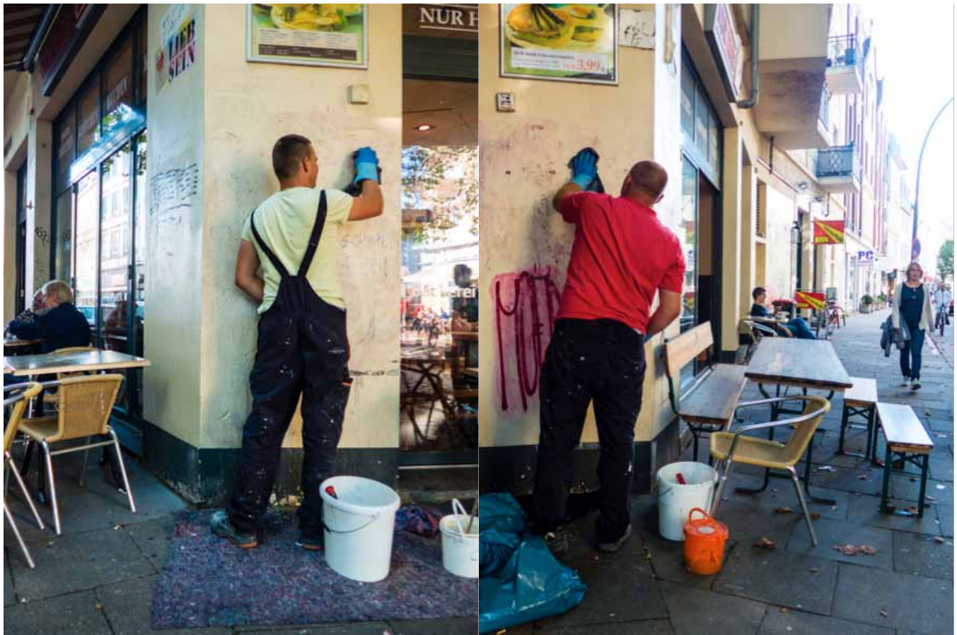
Fig. 7 - Chemical-based graffiti removal in a public area. Hamburg, Germany. 2016. Photos by D. Huntington.
