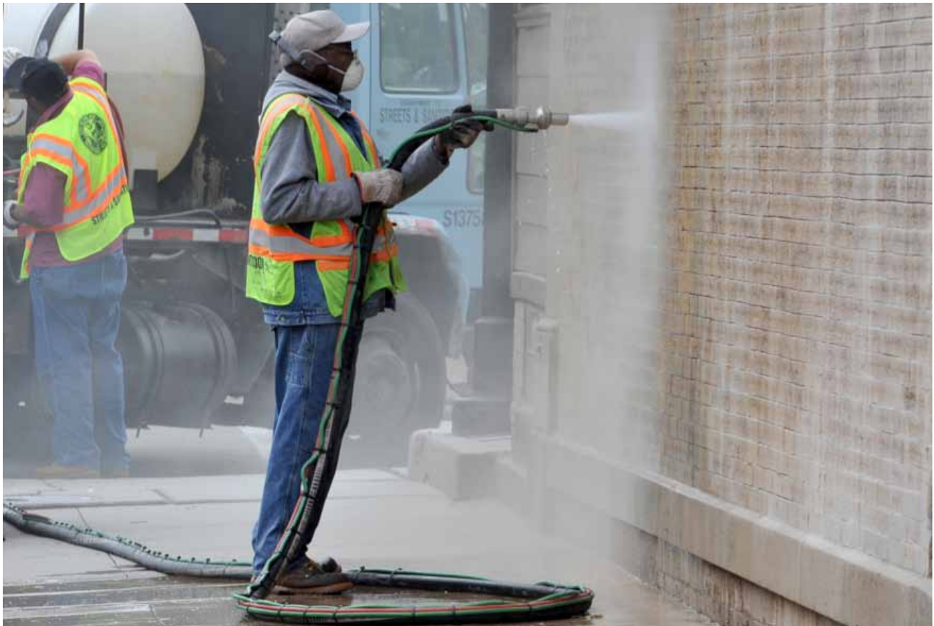
Fig.9 - The City of Chicago offers free graffiti removal on public and private property using pressure washer systems. Chicago, Illinois. 2013. Photo by A. Podgorski.
