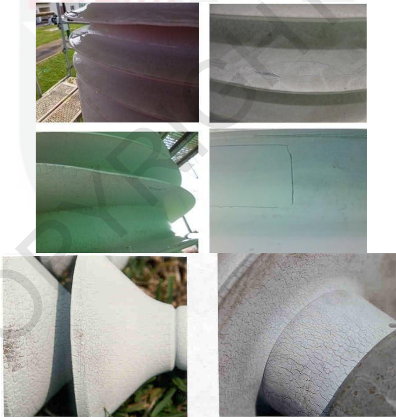
Figure 1.1 : Ageing and degradation of polymer housing [13]
