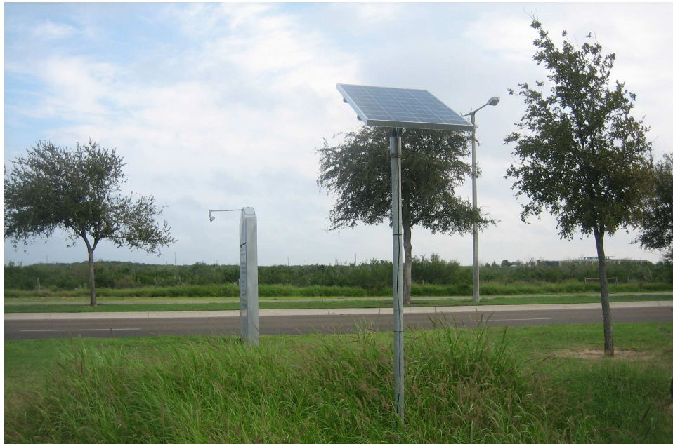
Figure 3: Solar Panel that Provides Lighting to Campus Signage
