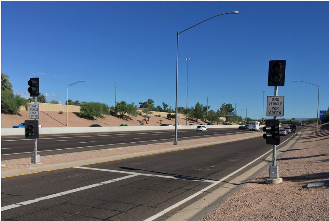
Figure B.1 Ramp meter image (used with permission from the Arizona Department of Transportation (ADOT, 2017)). Site photographed is along Arizona State Route 51 in the Phoenix area.
