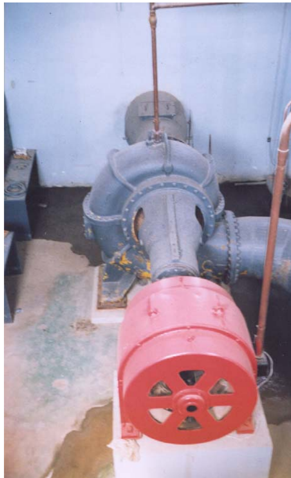
EXHIBIT C3. One 95-cfs Pump with Motor, Brownsville Irrigation District Rio Grande diversion pumping station, 2003.
