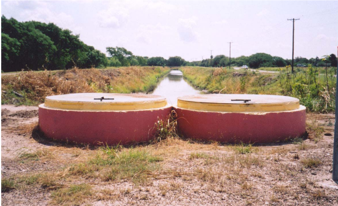
EXHIBIT C5. Two 52-inch Pipes Housing the Flow Meters, 2003. (Note: the Main Canal is located in the background).
