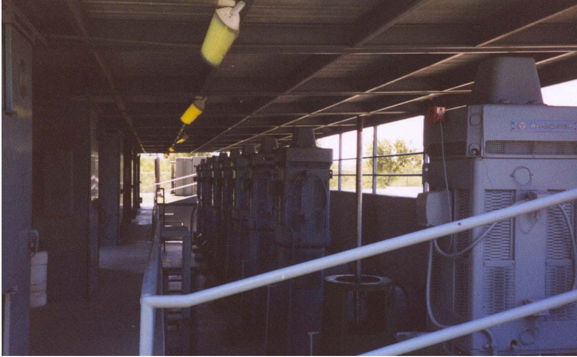
EXHIBIT C3. Internal View of the HCID2 Pump House, 2003 (Stubbs).
