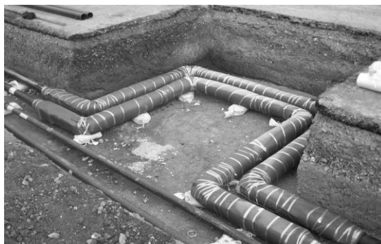
Figure 1. A thermal dilatation compensator in a pipeline [2]
