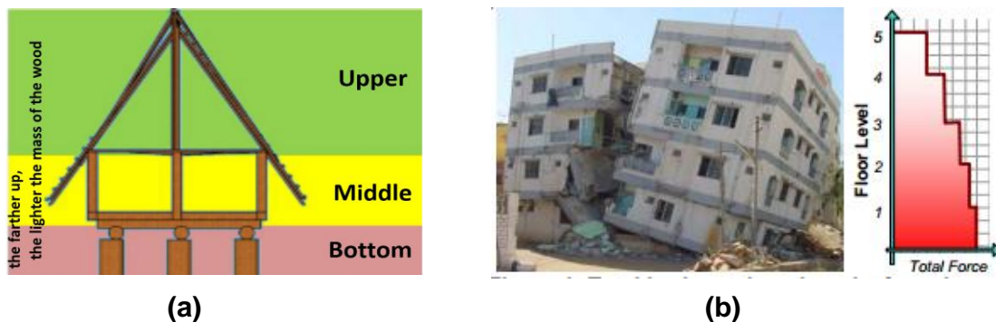
Figure 6. (a) Structure of Basemah House (modified from Rinaldi et al., 2015) and (b) Destroyed buiding Caused by Earthquake (Murty, 2005)
