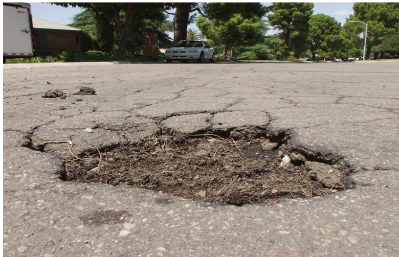
Figure 1.1. A pothole caused by fatigue failure (Source: dot.ci.tucson.az.us/streets/normal.htm )
