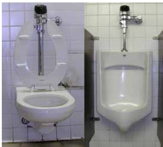
Figure 4. Automatic low-consumption water closet and urinal
