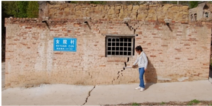
Figure 17 Case study of wall cracks.
