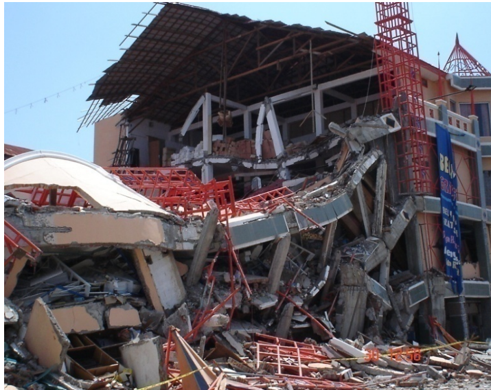
Figure 1 Buildings collapsed during the earthquake in Banda Aceh, 26th of December, 2004.
