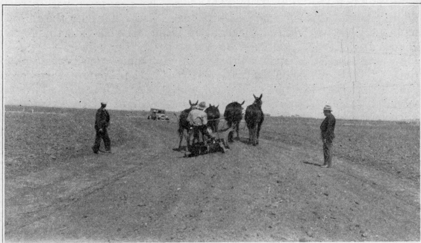
Fig. 23. A broad-base terrace under construction. This terrace is 24 feet wide at the base and is two feet high. Crops can be grown on top of this terrace and it can be planted and cultivated with two-row implements.
