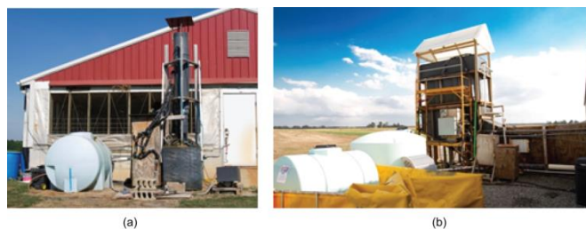
Figure 2 Actual photographs of scrubbers installed on the exhaust fan of (a) a deep-pit swine facility and (b) a poultry manure composting facility.
