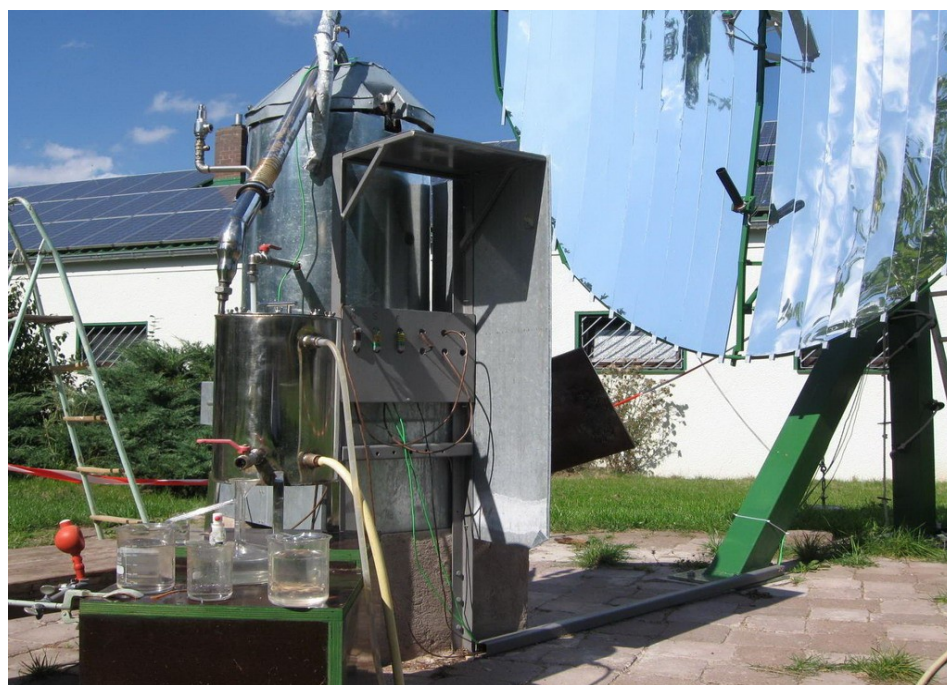
Figure 2. Solar distillation system for essential oils extraction using Scheffler reflector
