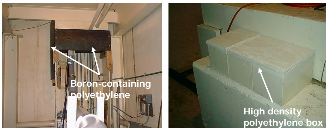
Fig. 2.14. Boron-containing polyethylene panel and portable wooden box for minimizing neutron streaming through the penetration and the concrete door.
