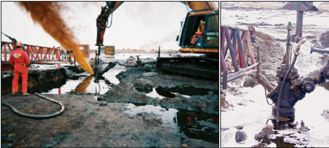
Fig. 5.4 – Dual stinger operation – Left: Stinging into casing valve, and pumping down stinger in tubing. Right: Post-sting and kill operation. 11
