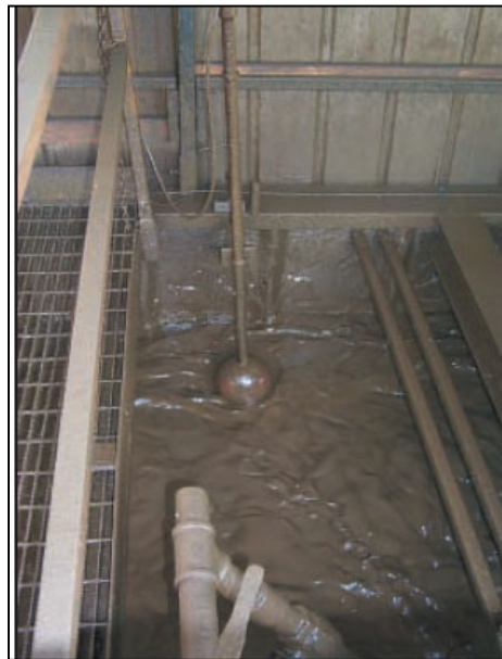
Fig. 3.3 – Float type pit level sensor. 29
