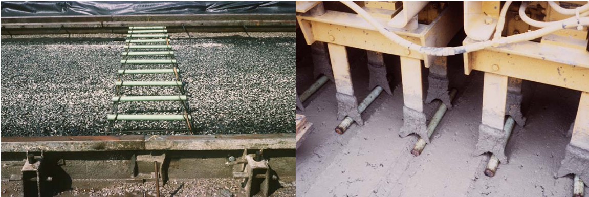
Figure 2-4 (Left) Dowel baskets in place prior to paving, (Right) Dowel bar inserter in operation.
