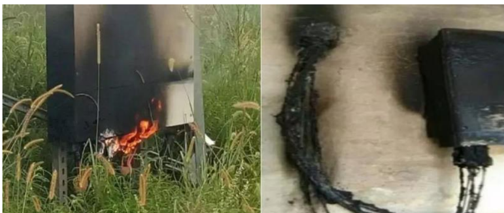
Fig. 2-7. Damaged combiner box by fire [32]
