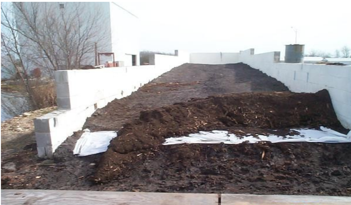
Figure 5.2 Failure of the berm on clay soil due to displacement.
