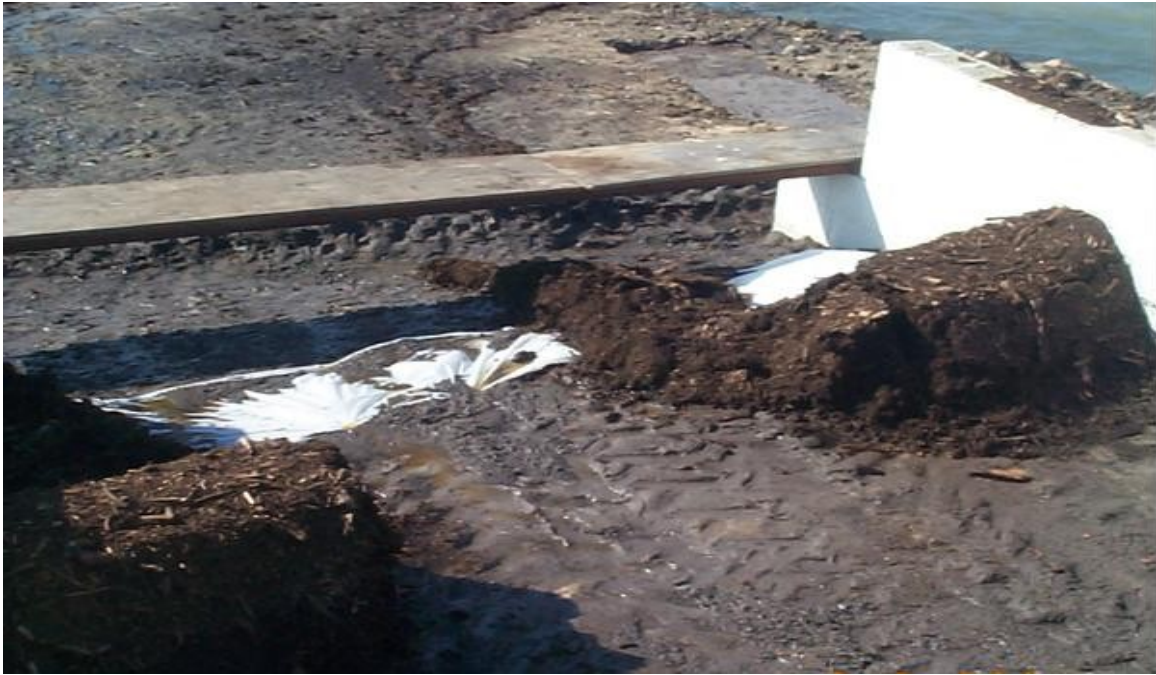
Figure 5.3 Lack of friction between clay soil and berm leading to failure by displacement.
