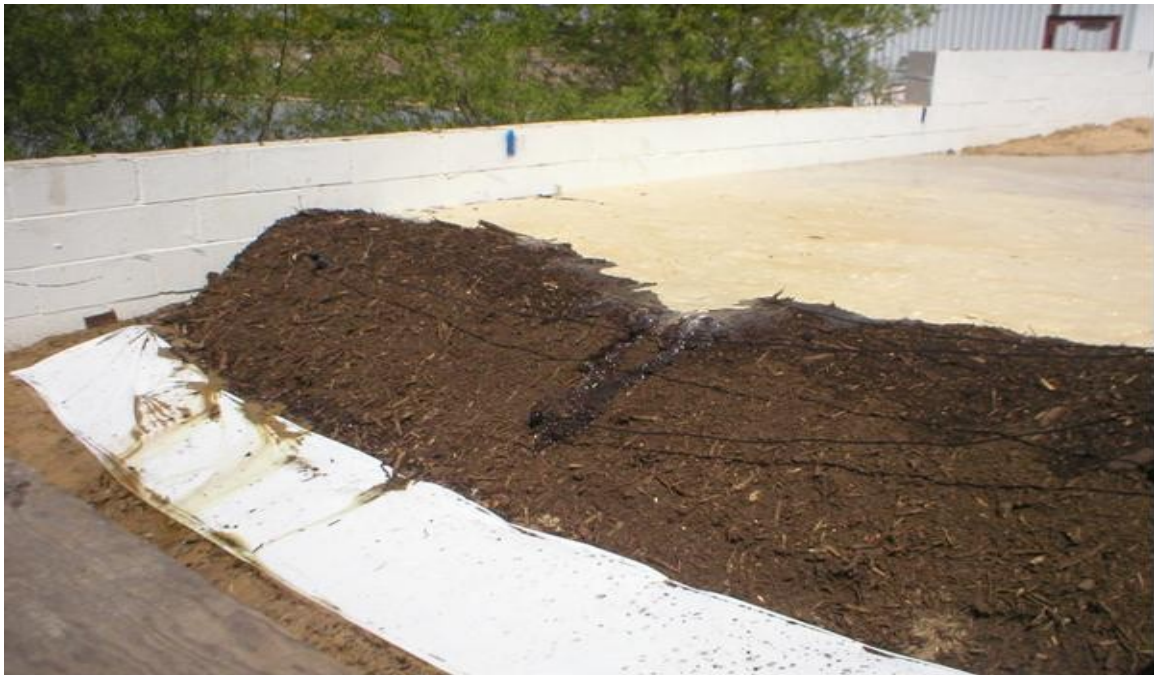
Figure 5.6 Compaction of the berm leading to overtopping with very little infiltration.
