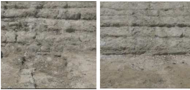
Figure 9. Pit created at the toe of the downstream slope after overflow testing on the untreated soils (left) and comparison with limited erosion on the lime-treated soil (right); picture taken after 17 hours testing.
