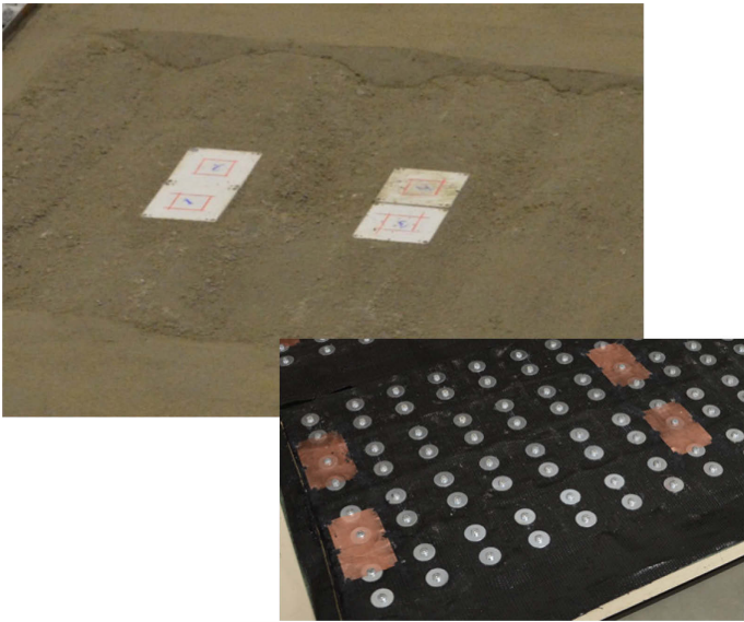
Figure 5. Copper plates are attached to the block mattress in order to measure the displacement of the mattress with the displacement sensors, which are incorporated in the floor.
