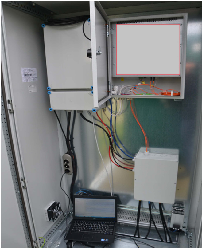
Figure 3. DTS instrument from APSensing and auxiliary equipment for the heating cycles. The system is remotely controlled.
