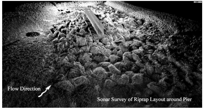
Figure 4 Multibeam sonar scan of the installed riprap apron at Pier 3 of the Middle Fork Feather River Bridge (BlueView Teledyne Marine)
