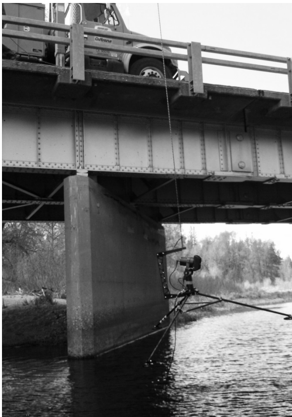
Figure 3 Deployment of the Multibeam Profiler Sonar at the Middle Fork Feather River Bridge.
