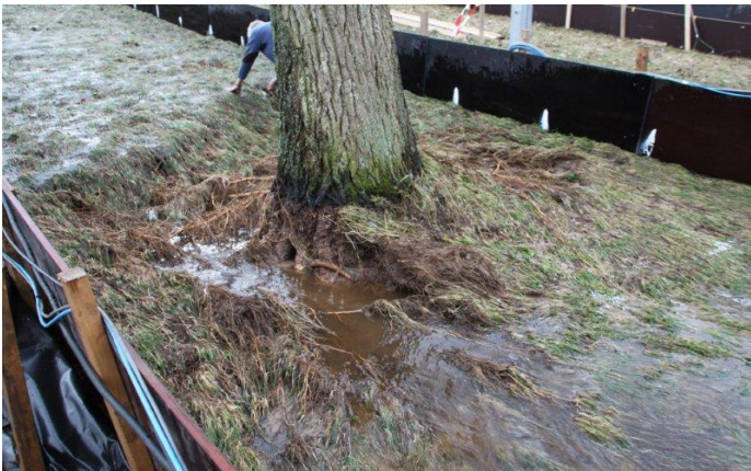
Figure 3.6 Erosion at tree (halfway the inner slope of the dike)
