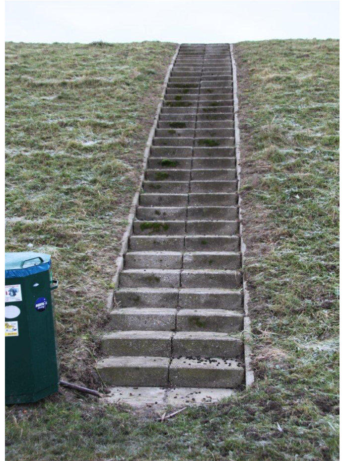
Figure 2.2 Patchy turf; Tholen, Section 2, Stair (before testing)
