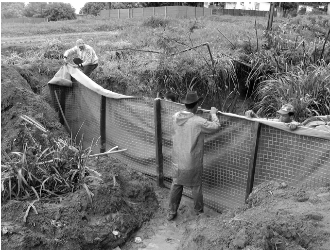
Figure 2. Silt fence in erosion channel (courtesy R.J.C.Farias).
