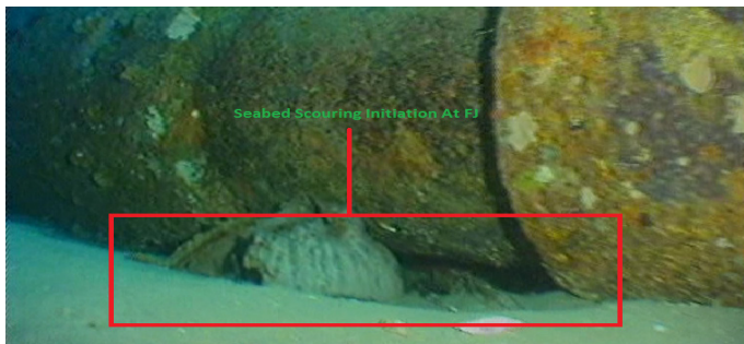
Figure 3 Field Observation of Scour Initiation at a Field Joint Location
