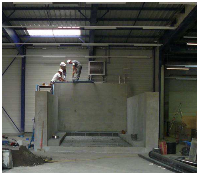
Figure 6. Construction of the reinforced concrete structure for testing the large scale models.
