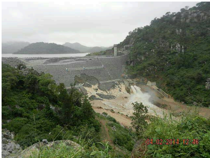
Figure 28. Backward erosion during the construction of the Mokwe Mukorsi CFRD dam
