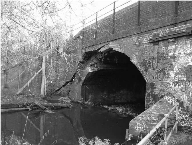
Figure 1. Upstream face of Bridge RDG1 48 showing failed arch following debris blockage (after RAIB 2010).
