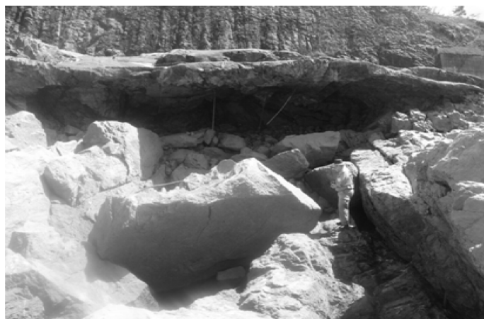
Figure 9. Large scour hole in spillway following 2010-2011 flood event at Boondooma Dam
