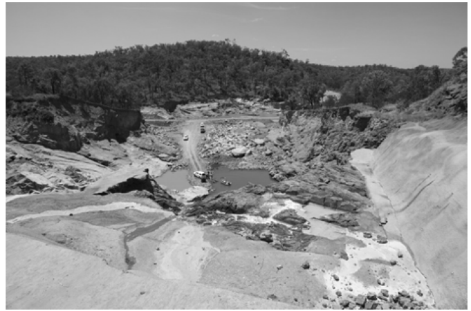
Figure 10. Large scour hole in downstream part of spillway following 2010-2011 flood event at Boondooma Dam
