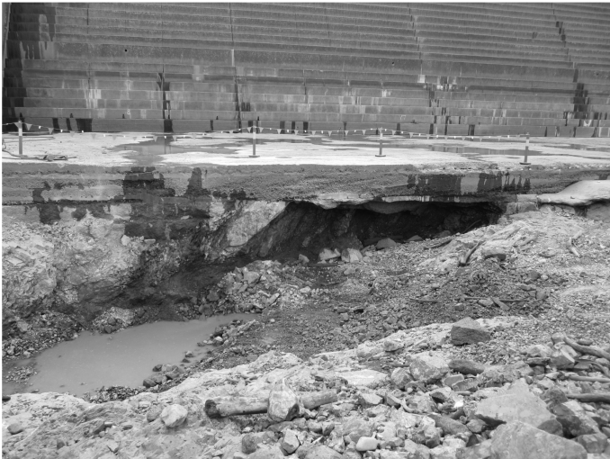
Figure 6. Apron undermining following 2013 flood
