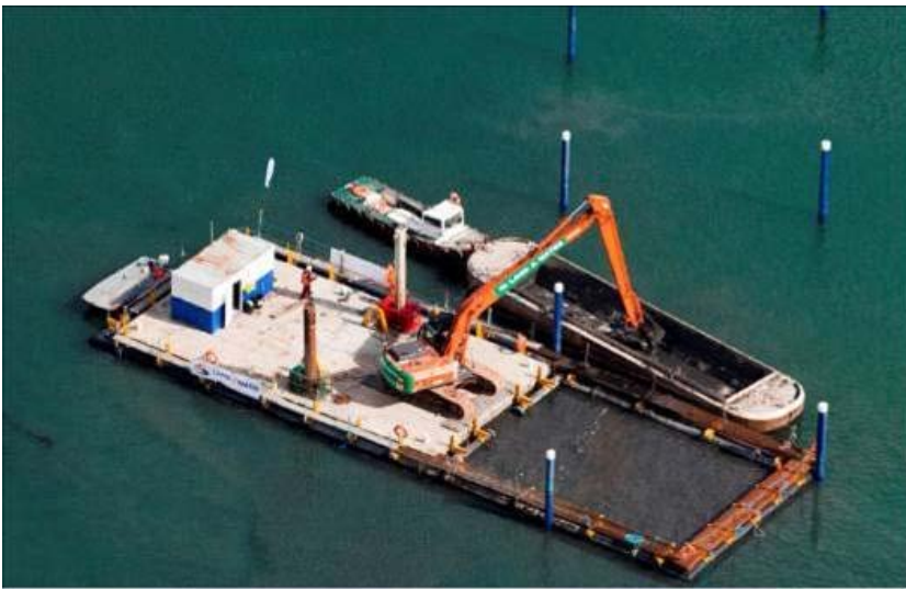
Figure 1: Photograph of an enclosed framed silt curtain
