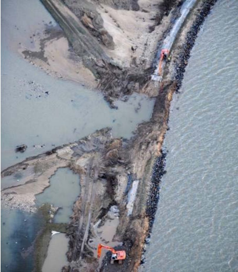
Figure 4: Aerial view of the damage to a section of coastal flood defences in Vendée
