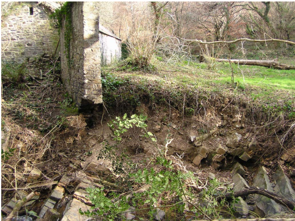
Plate 3.19 Erosion of bank under stone building wall
