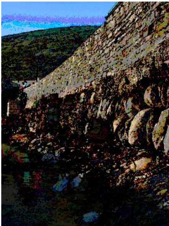
Plate 7.2 Erosion and undermining of Pengold Stream and the main road bridges
