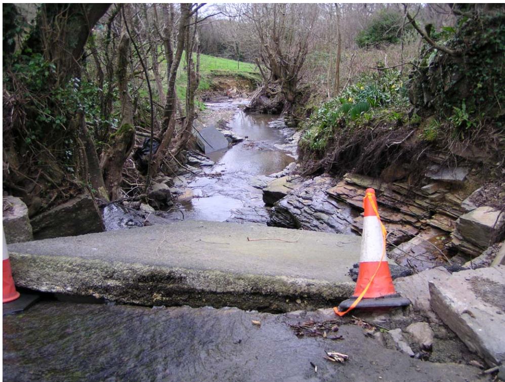
Plate 3.21 Erosion at Lansweden ford
