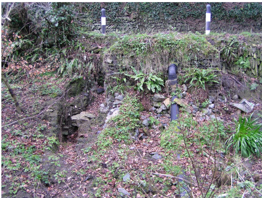
Plate 3.10 Overland runoff from roads causing erosion
