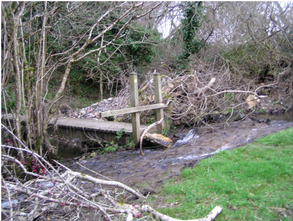
Plate 3.16 Avulsion at footbridge on Tresparrett Stream
