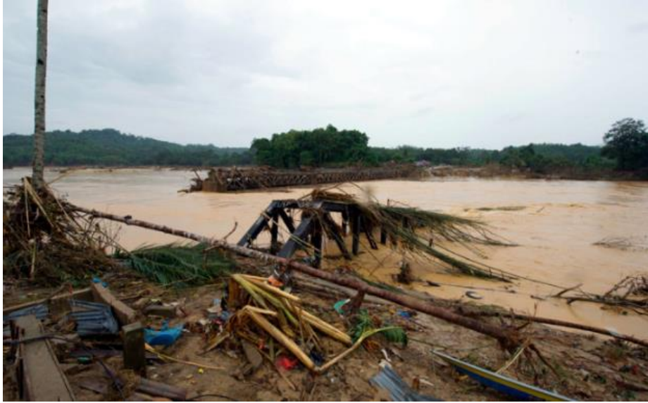
Fig. 3. Washway of railway tracks occurred in Malaysia East Coast Line railway bridge, which cross Nenggiri River in Kemubu, Kelantan had totally lost due to massive flood in December 2014. (Courtesy: Malaysian Department of Public Works)
