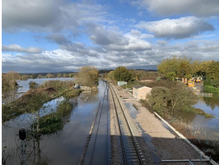
Fig. 1. A flooded turnout. The picture courtesy of East Midlands Railways.
