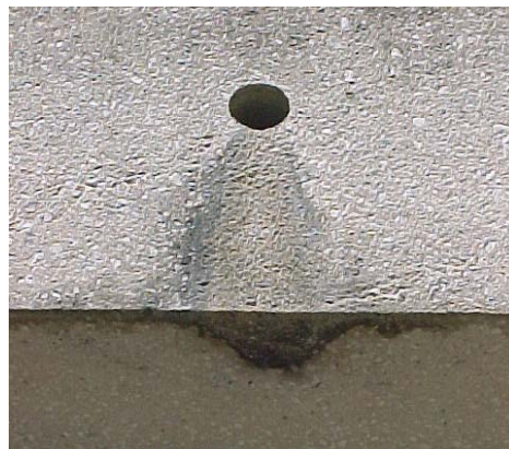
Fig. 19. A staining pattern on concrete caused by water flow.
