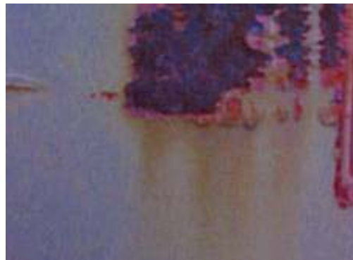
Fig. 2. Rust stained paint.
