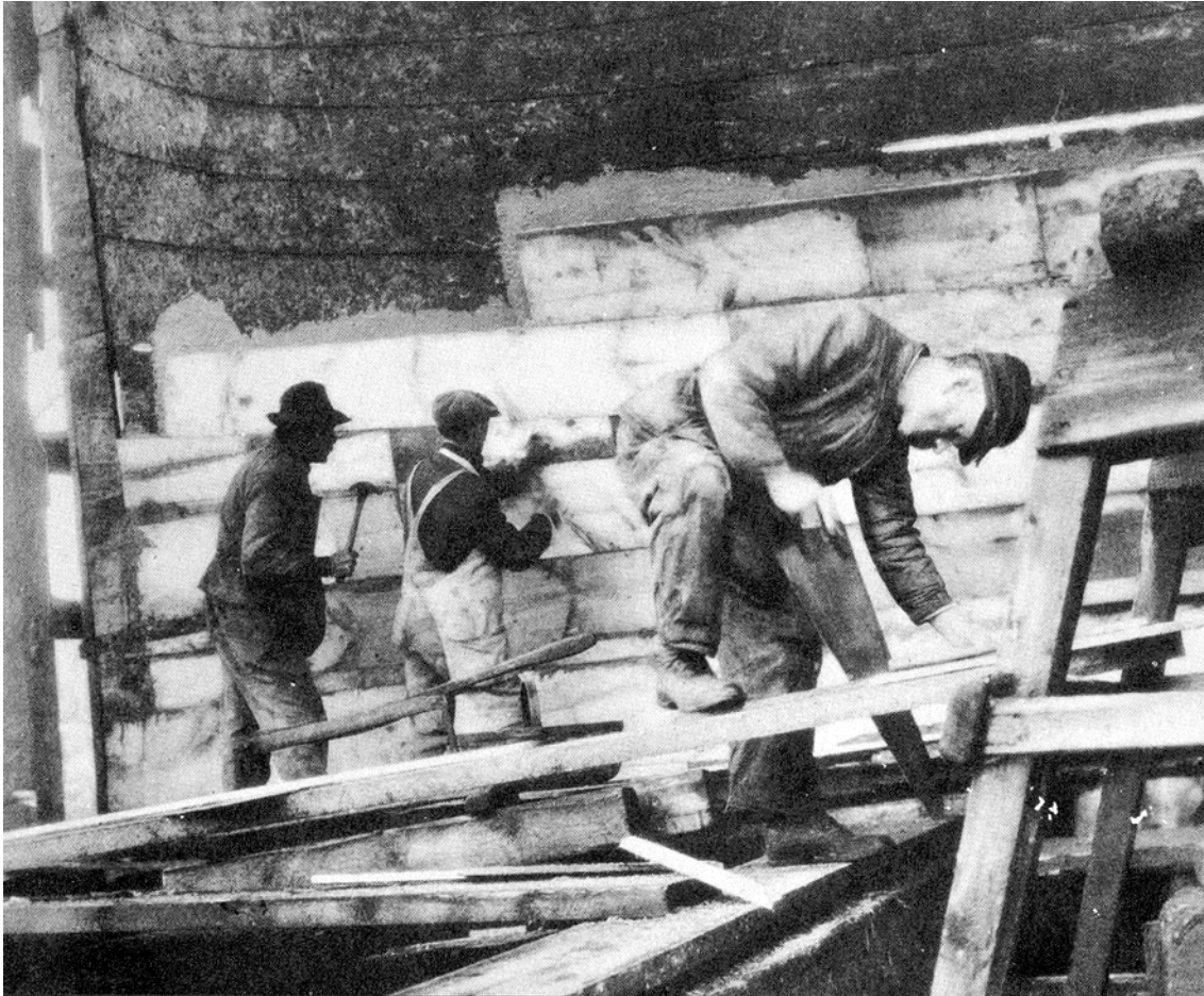
Figure 36. Carpenters applying pine sheathing before the application of metallic sheathing (From Church 1938, Figure 17).
