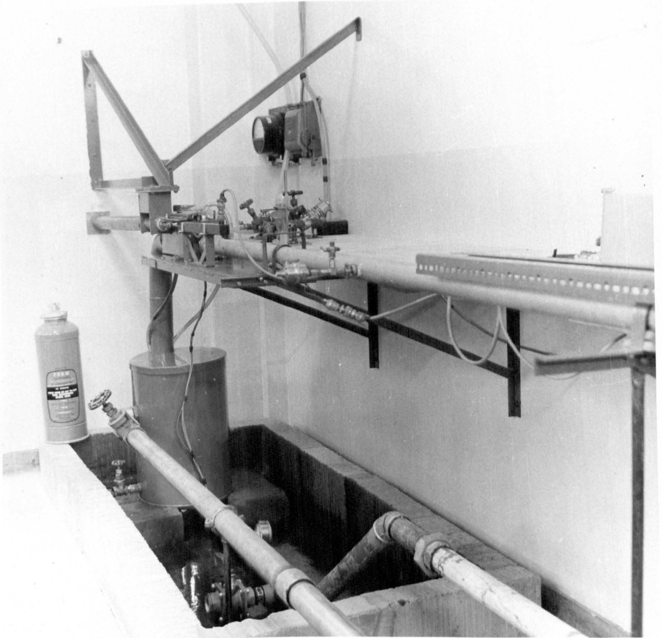
Fig. 21 Valve end of pipeline configuration 1, illustrating the independently mounted valve closing ram and the submerged fuel pump.
