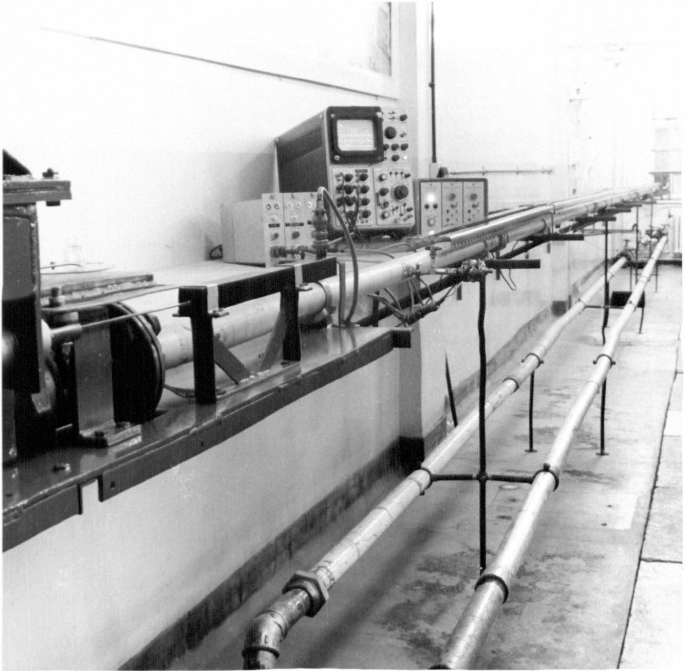
Fig. 22 View upstream from the valve in pipeline configuration 1, illustrating the pipe support brackets.
