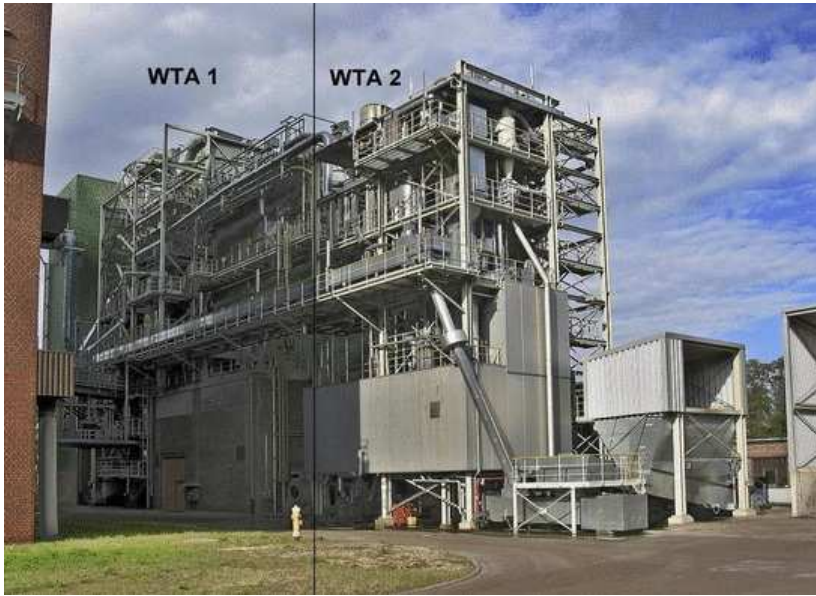
Fig. 19 Photo of the WTA 1 plant (left part) and WTA 2 plant (right part) at Frechen.
