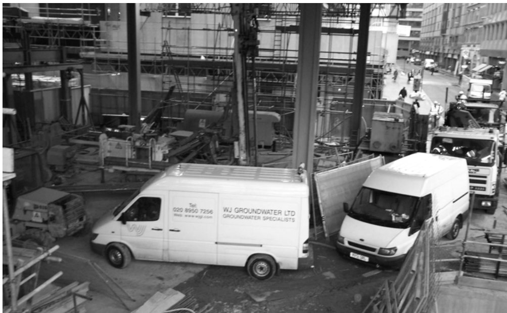
Figure 4 Congested site access with 14 tonne drilling rig operating on ground floor slab.
