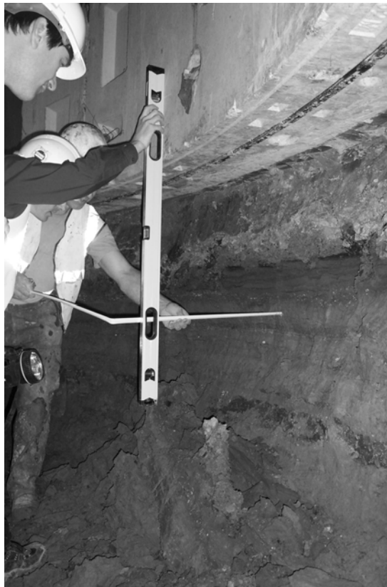
Figure 14 Silty sand slumping from the excavated face during ring build in water bearing layer in Upper Lambeth Group
